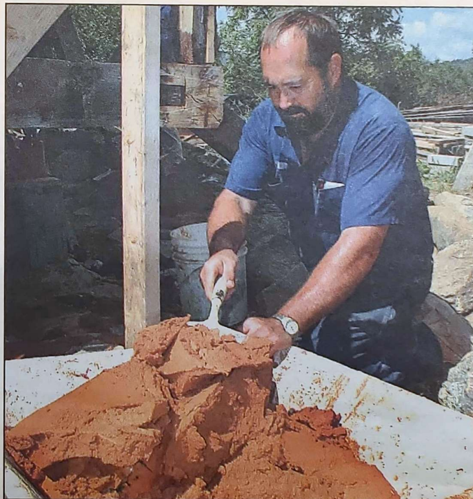
Edward Ashby mixes a clay/lime-putty mortar while shoring up the foundation of the circa-1763 boyhood home of Chief Justice John Marshall.
