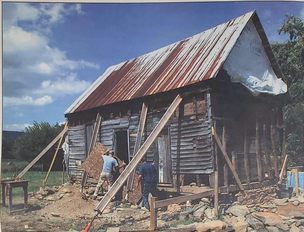
Mike Adams, left, and Edward Ashby work on stabilizing the circa-1763 boyhood home of Chief Justice John Marshall. The home is located in Markham.
